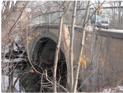
Mystic Valley Parkway Bridge in need of repair. ~Photo by Bobbie Toner
